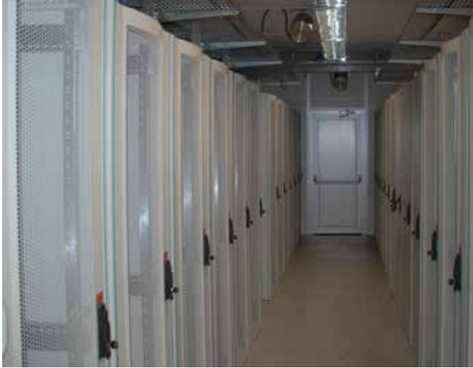
MED-NAUTILUS TELECOMMUNICATION CO.INC. DATA CENTER
